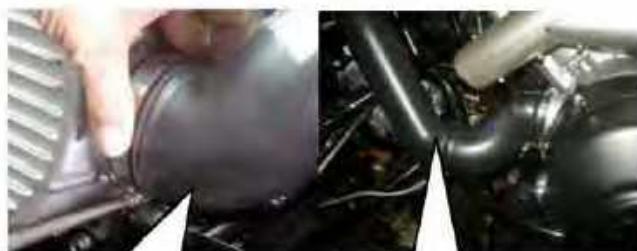
cooling outlet duct
